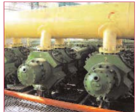
Above, a six cylinder reciprocating compressor, used to compress natural gas for piping over long distances. All six cylinders must remain healthy to maintain the required pressure and flow rate
